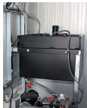
Serbatoio gasolio Fuel tank
