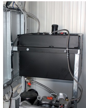
Serbatoio gasolio Fuel tank
